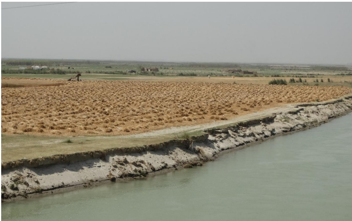
Image 55 : Bank Erosion At Balawali
