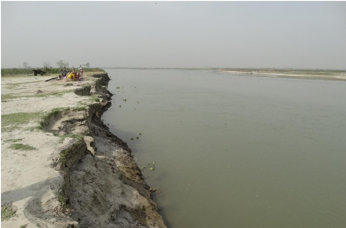
Image 54 : Lateral Bank Erosion At Daranagar Ganj
